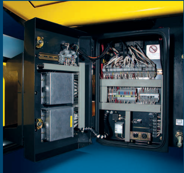
Central electrics: clearly laid out, highly reliable, simple to repair.
