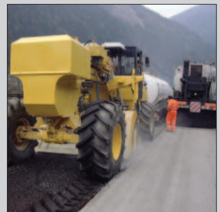
Additional possible applications in recycling by injection of bitumen emulsion or foam bitumen.
